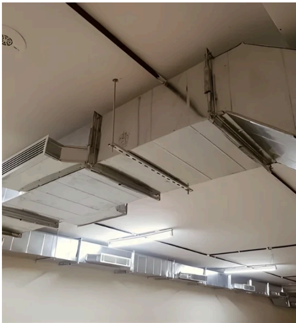
Mechanical Ventilation System
